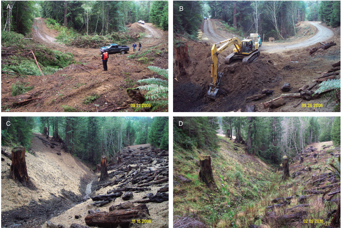
Plate 9 (Figure 5.3) Complete removal of a forest road in Salmon Creek, Humboldt County, California: (A) before; (B) during; (C) immediately after; and (D) 3 years after removal of stream crossing and road fill. Note that the stream side-slopes were laid back to a stable grade that mimics natural hillslope topography and all bare slopes were mulched with rice straw. The excavated stream crossing has also been sloped to a stable angle and mulched to control surface erosion. Photos courtesy of California Department of Fish and Game Fisheries, Bureau of Land Management, Pacific Coast Fish, Wildlife & Wetlands Restoration Association, and Pacific Watershed Associates.
