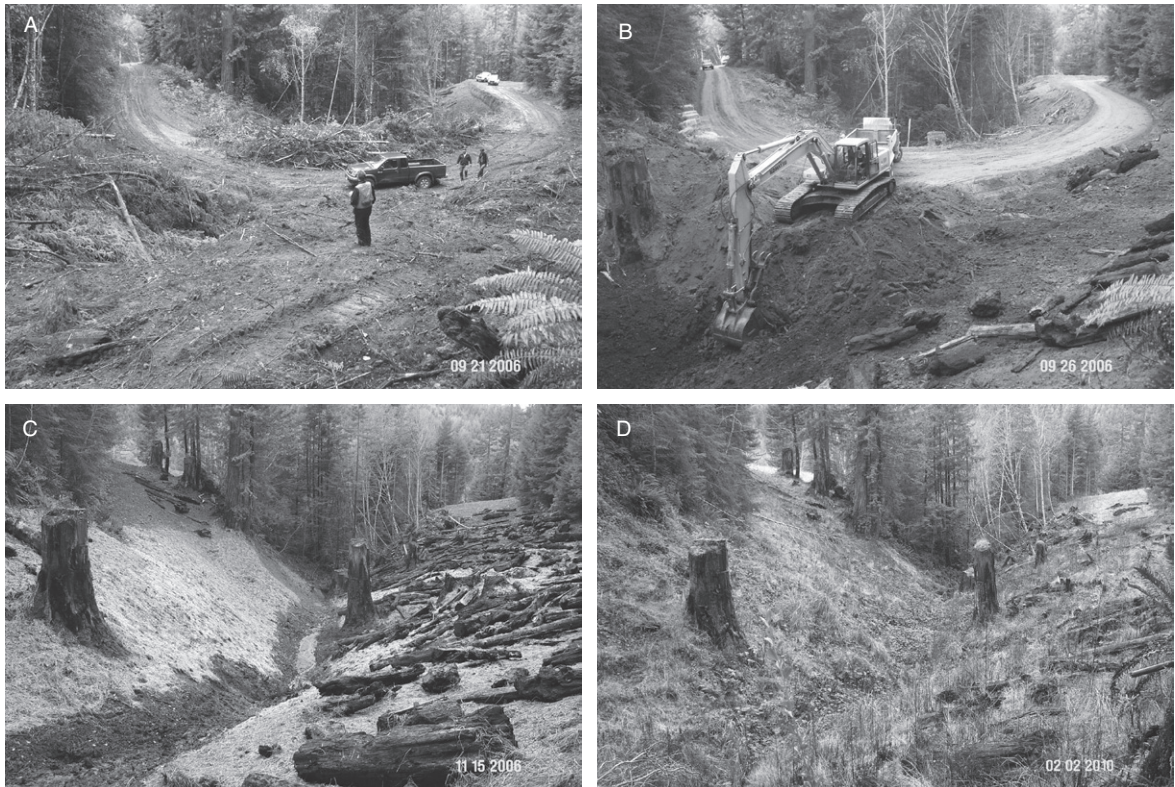
Figure 5.3 Complete removal of a forest road in Salmon Creek, Humboldt County, California: (A) before; (B) during; (C) immediately after; and (D) 3 years after removal of stream crossing and road fill. Note that the stream side-slopes were laid back to a stable grade that mimics natural hillslope topography and all bare slopes were mulched with rice straw. The excavated stream crossing has also been sloped to a stable angle and mulched to control surface erosion. Photos courtesy of California Department of Fish and Game Fisheries, Bureau of Land Management, Pacific Coast Fish, Wildlife & Wetlands Restoration Association, and Pacific Watershed Associates. (See Colour Plate 9)
