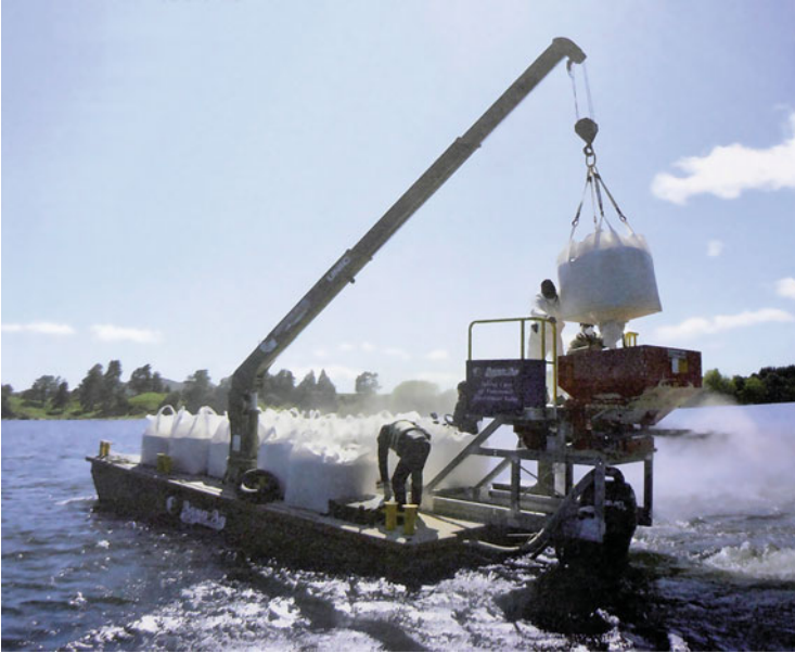
Fig. 7.15 Applying granular Aqual-P ® using a fertiliser spreader on a barge [photo Andy Bruere, BOPRC]
