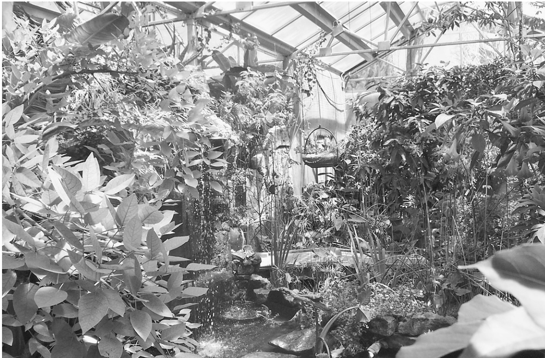
Figure 4.5 Treated water from the Living Machine enters an indoor display pond at El Monte Sagrado resort in Taos, New Mexico. (Photo courtesy of Worrell Water Technologies.)
